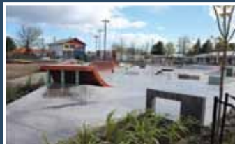
CAST-IN-PLACE, SPECIAL FINISHES Under 5000 SF – 2nd Place Project: William Nelson Skate Park Contractor: Angus McMillan Concrete, Ltd.
